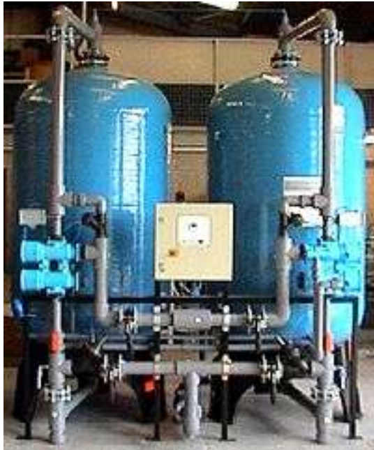
Ion exchange plant
